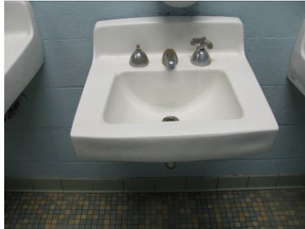
Typical Lavatory Missing HW Handle
