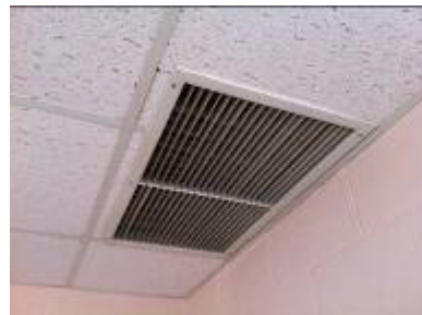
Typical Classroom Exhaust Register
