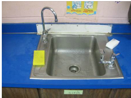
Typical CR Sink Missing HW Handle
