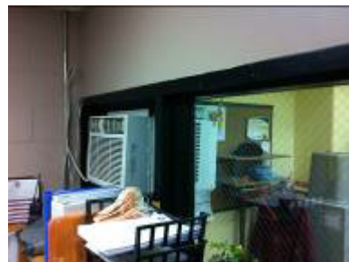
Typical Window Air Conditioner at Interior Space
