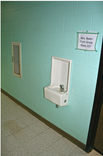
Typical Signage & Drinking Fountain
