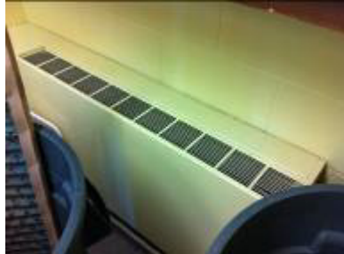
Typical cabinet Unit Heater
