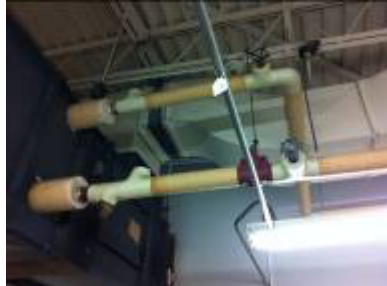
Typical Hot Water Piping at AHU
