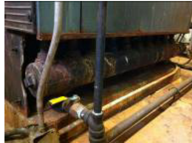
Main Boiler Barrel Condition
