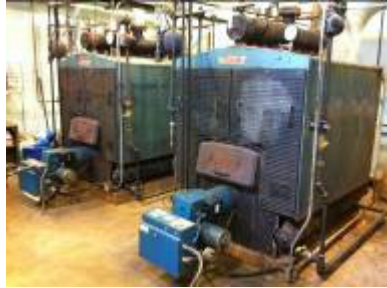
HW Boiler Plant
