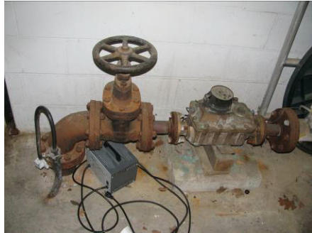
Water Service and Meter
