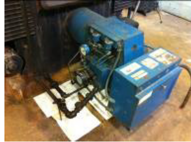
Fuel Oil Burner
