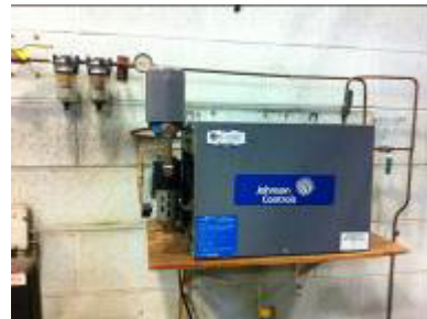
Refrigerant Air Dryer
