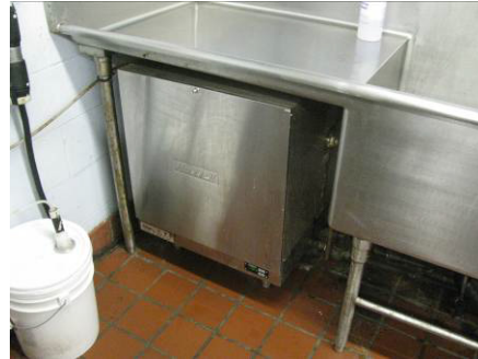
Kitchen Electric Booster Heater
