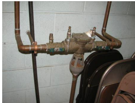
Boiler Make-up Backflow Preventer
