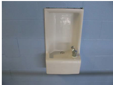
Typical Drinking Fountain
