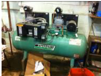
Pneumatic Control Air Compressor
