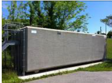
Outdoor 10,000 Gallon Oil Tank
