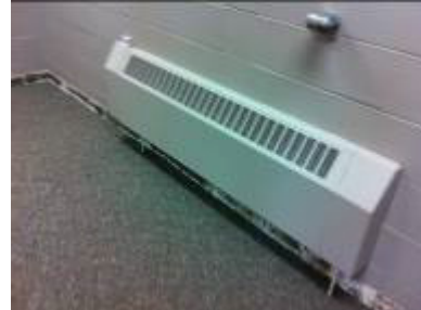
Typical Bathroom Fintube
