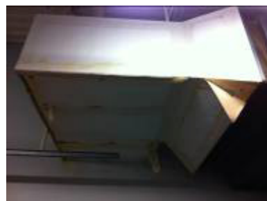
Typical Duct Insulation
