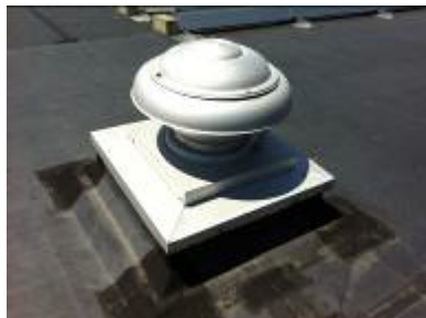
Typical Roof Mounted Exhaust Fan
