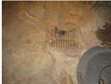
Boiler Room Floor Drain
