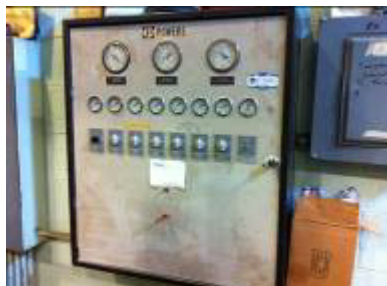
Powers Control Panel
